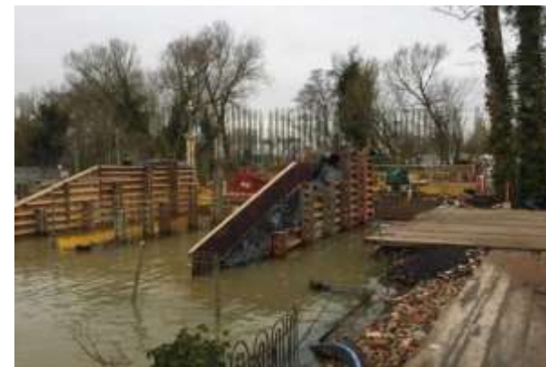
Figure 9: Flooded cofferdam in February
